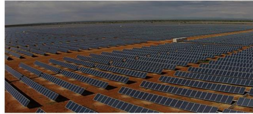
Fig.6. Benban solar park in Egypt.
